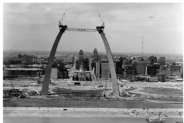
Construction of the Gateway Arch in St. Louis, dated July 8, 1965. From the Missouri Department of Transportation Collection.
