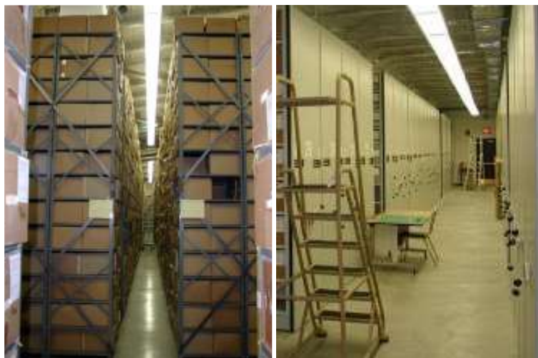
Lighting over fixed shelves (left) and over mobile shelves (right).
