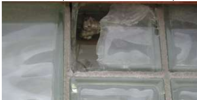
An example of a broken building envelope, where wasps have made a nest in a broken window.
